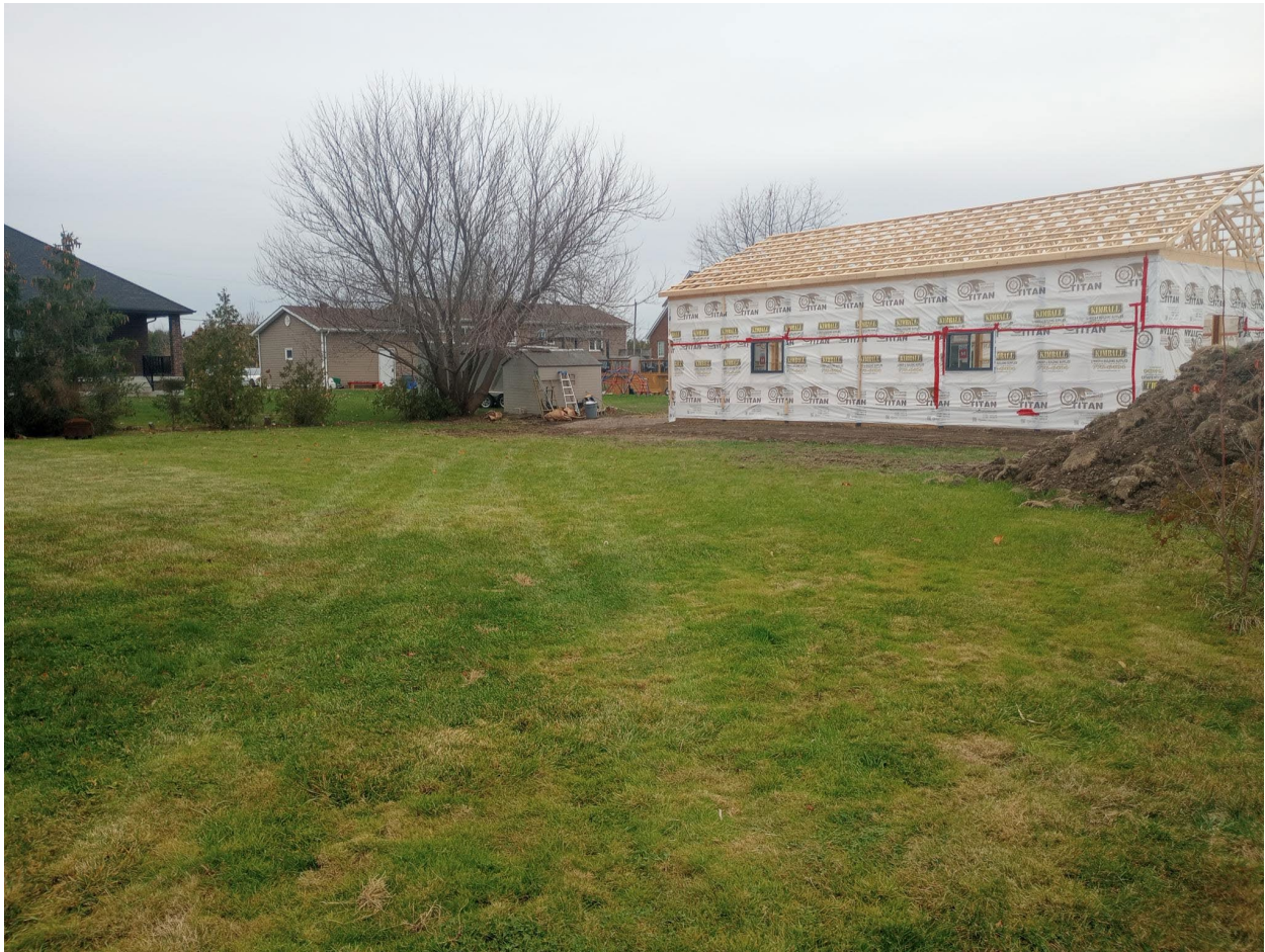
Picture of lot addition land looking northwest towards 2368 Lakeshore Road 223 and 2364 Lakeshore Road 223. Building under construction located in the rear yard of 2364 Lakeshore Road 223 is visible in the photo.
