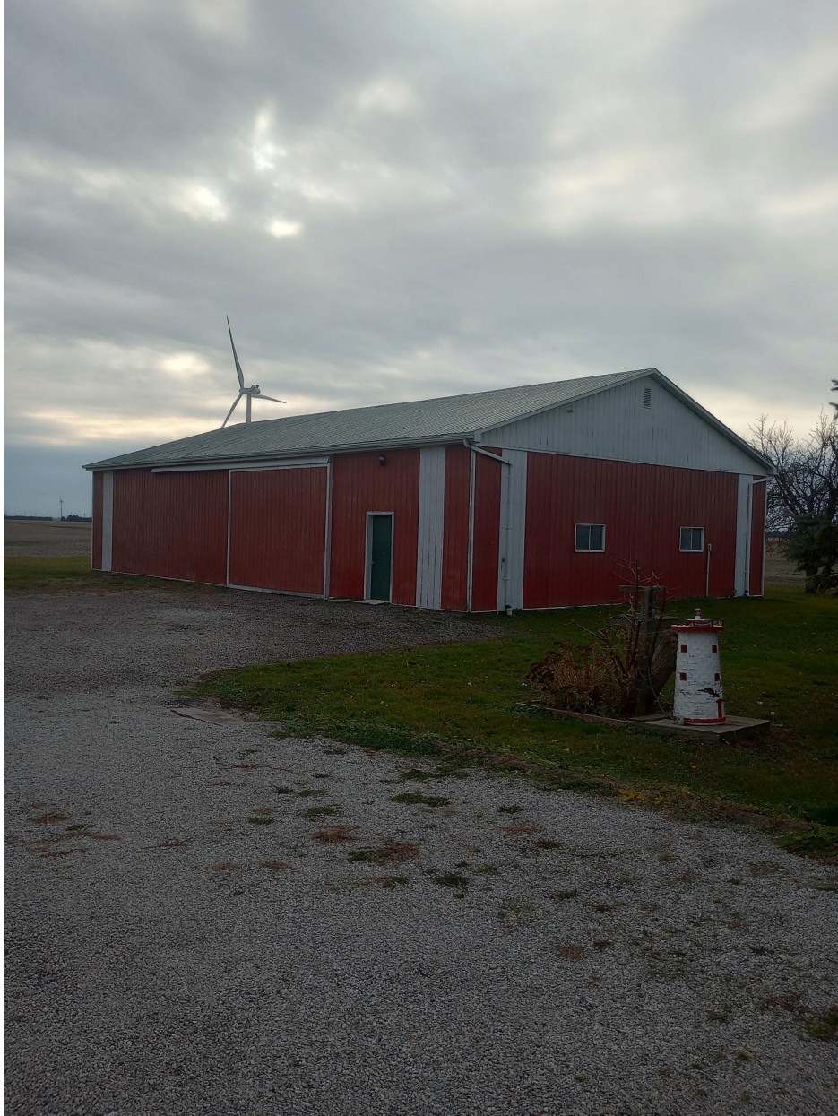
Looking southwest towards the accessory structure located near the southwest corner of the proposed severed lot
