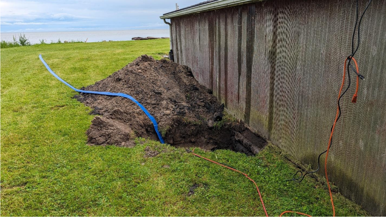
Figure 2 – Exposed foundation hole on the West side of the building (lean-to portion).
